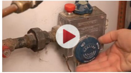
Adjusting Your Hot Water Tank (3:18)
